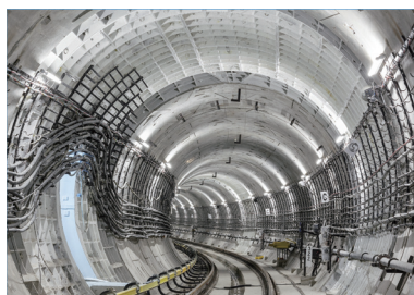
Environmental Monitoring of Rail Transit
